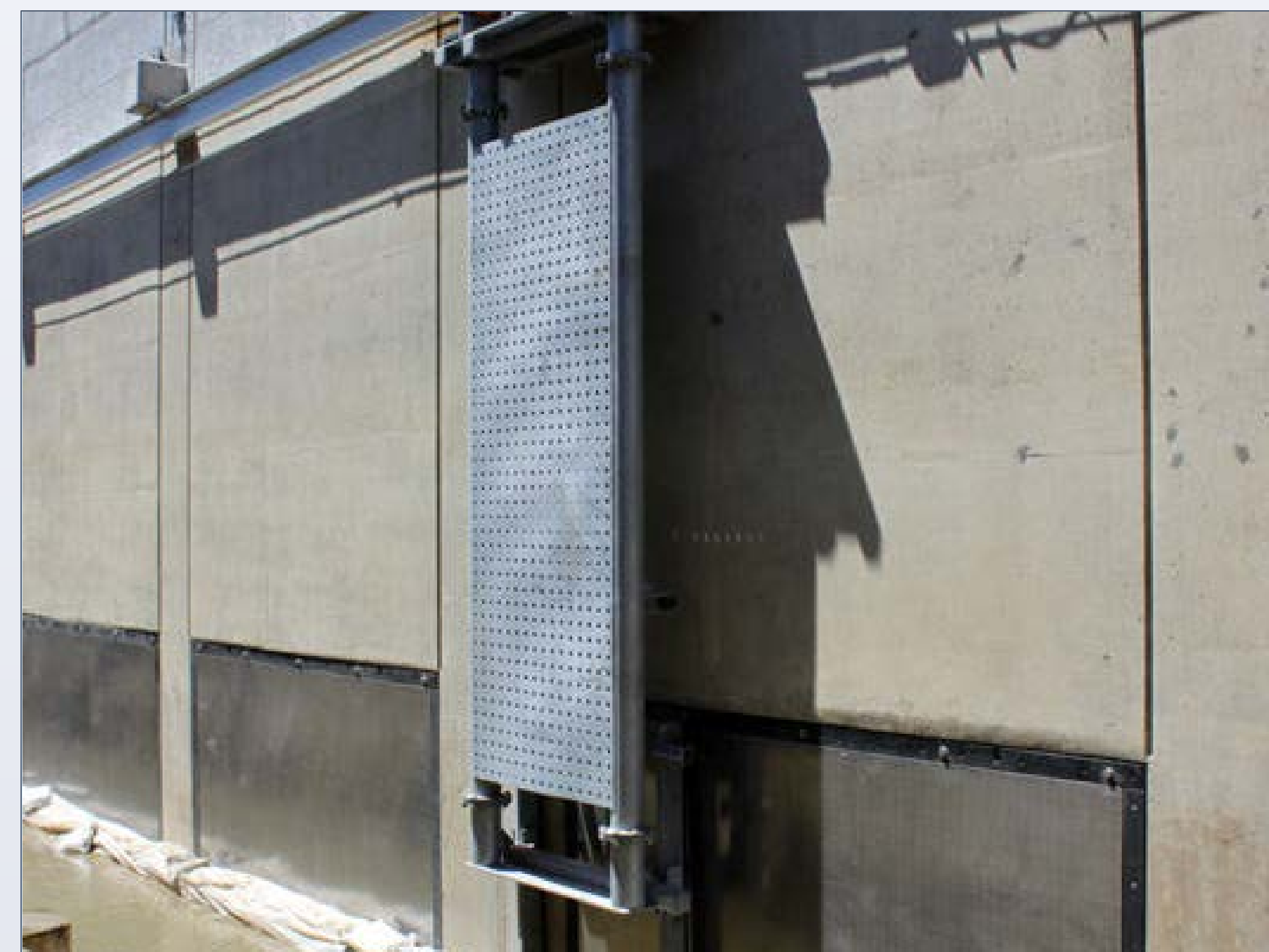
Fish Screens and Mechanical Cleaner
