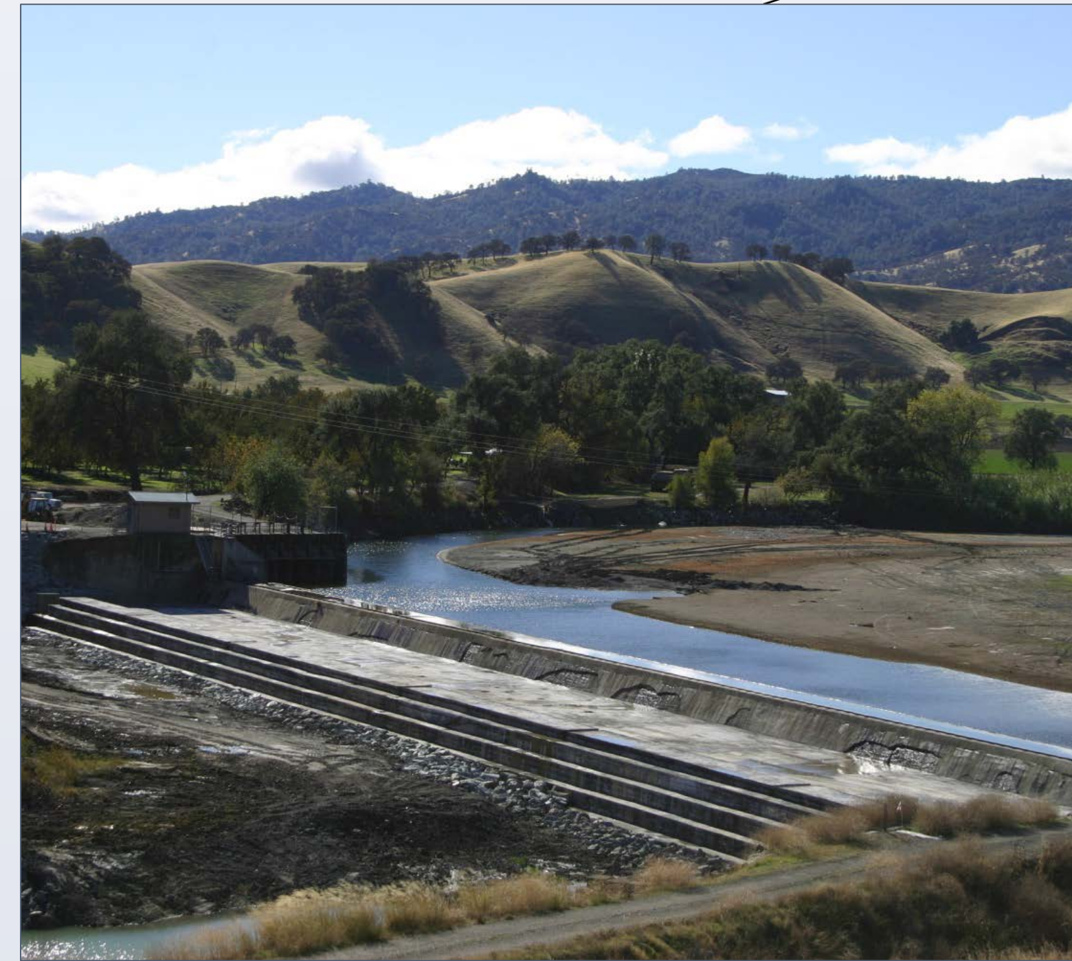
Capay Diversion Dam Apron Repair Yolo County Flood Control & Water Conservation District
