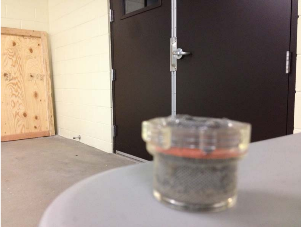
Photo #8: Clogged Basket Strainer
