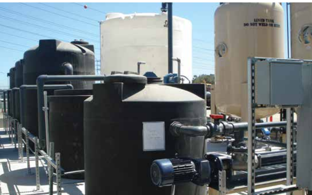
Photo caption: Demonstration facilities tested the potential of reduction/coagulation/filtration (RCF) water treatment technology for removal of hexavalent chromium.
